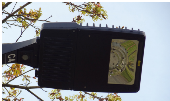
After: New LED luminaires offer better optical performance and light distribution
